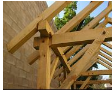
Here is a close up of the joint at the top of the stav showing how the sperre fits on the stavlaegje.
